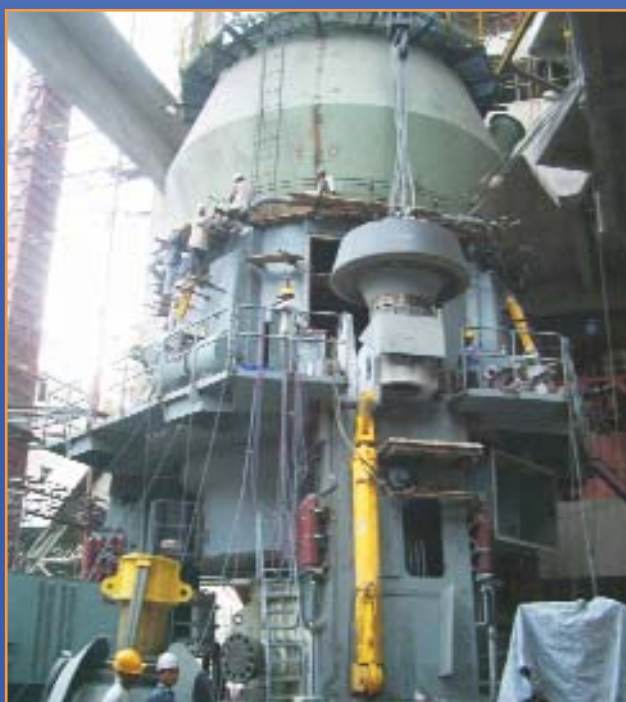
Figure 10. LM 56.3+3 in Rajgangpur plant of Orissa Cement, India.
