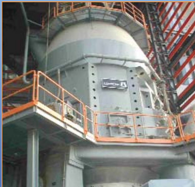
Figure 9. LM 46.2+2 in Ras-El-Ma plant of Holcim Maroc.
